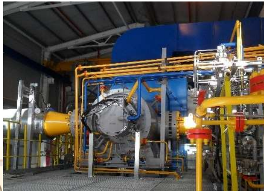
Natural Gas Pipeline Compressor
