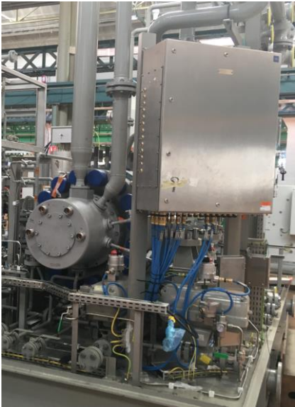
Junction Box Arrangement Cabling
