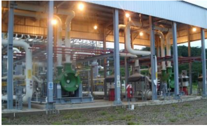
Figure 15 – Both compressors in Operation at site In Bolivia
