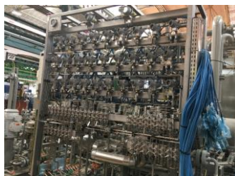
Figure 10 - DGS Monitoring Panel
