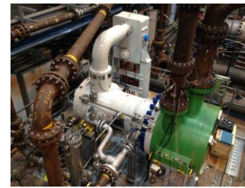
Figure 14 – ICML during Factory Testing
