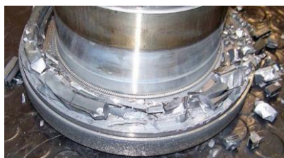
Figure 5 - Dry Gas Seal Catastrophic Failure
